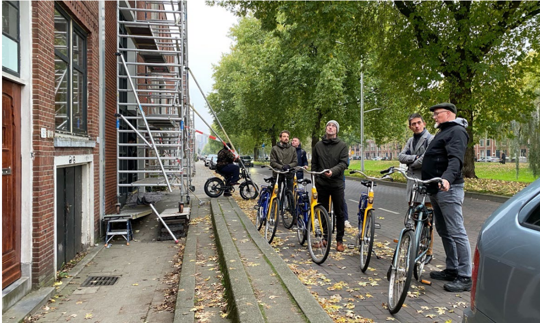
Expedition by the working group in Bloemhof, Rotterdam-Zuid. The houses have subsided compared to the street which used to be at the same level.
